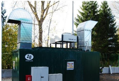
Combined heat and power plant
